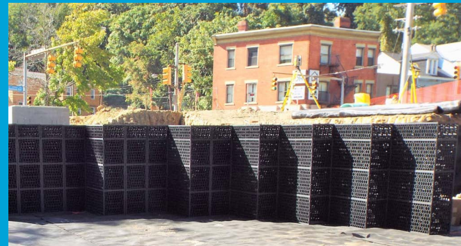
Partially installed R-Tanks at the bottom of the Centre and Herron Stormwater Project in the Hill District.
