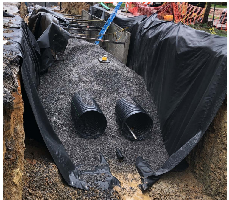
Layers of gravel and storage pipes will hold stormwater below the McPherson Boulevard median.
