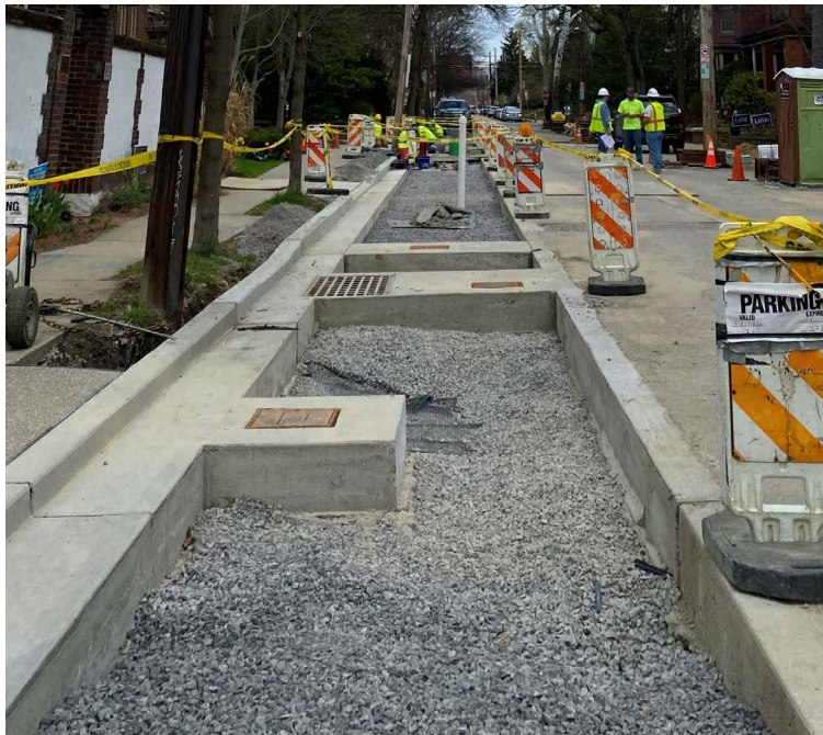
Permeable pavers will be installed over these layers of gravel and underground storage pipes on Howe Street.
