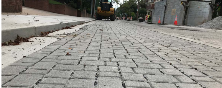
The stormwater fee will support the construction of new stormwater infrastructure in Pittsburgh.
