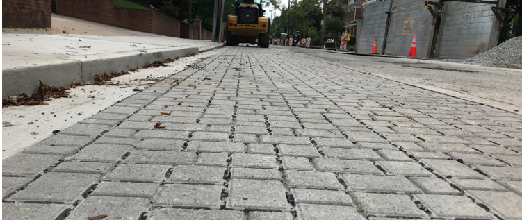
The stormwater fee will support the construction of new stormwater infrastructure in Pittsburgh.
